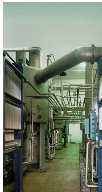
Installed Evaporation Plant
