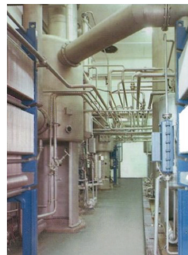
Installed Evaporation Plant
