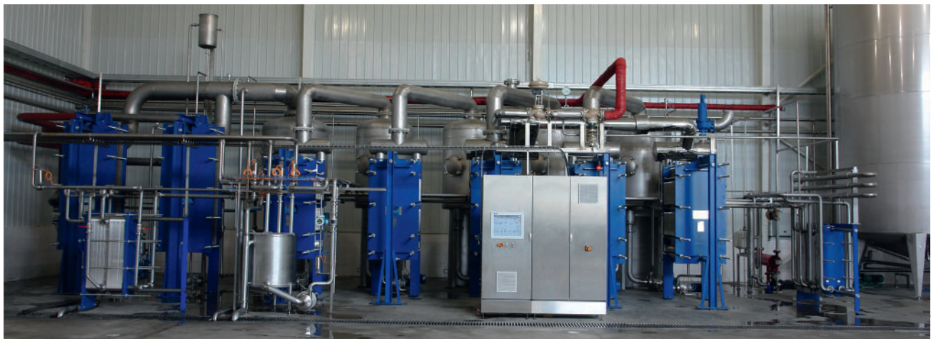
5-stage SIGMASTAR® 90V Evaporating Plant with thermal vapor compressor for apple juice - evaporating capacity 20,000 kg/h
