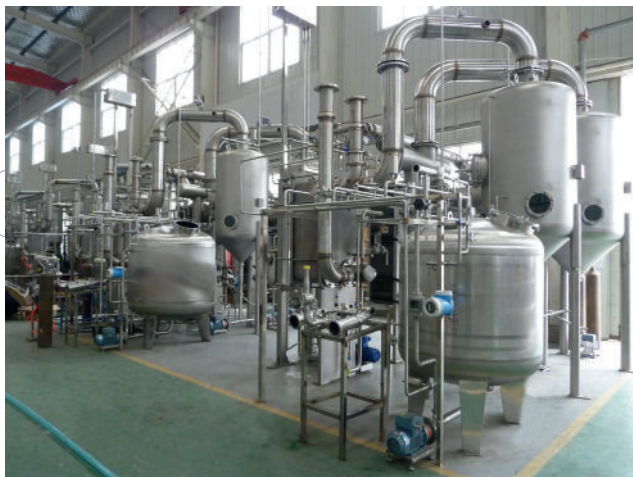
2-stage SIGMASTAR® 90V Evaporating Plant protein hydrolyzate - evaporating capacity 2,000 kg/h
