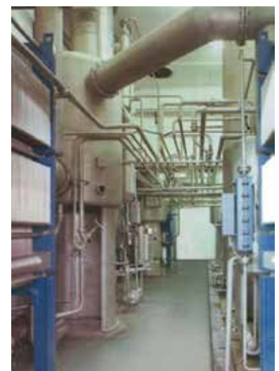
Installed Evaporation Plant
