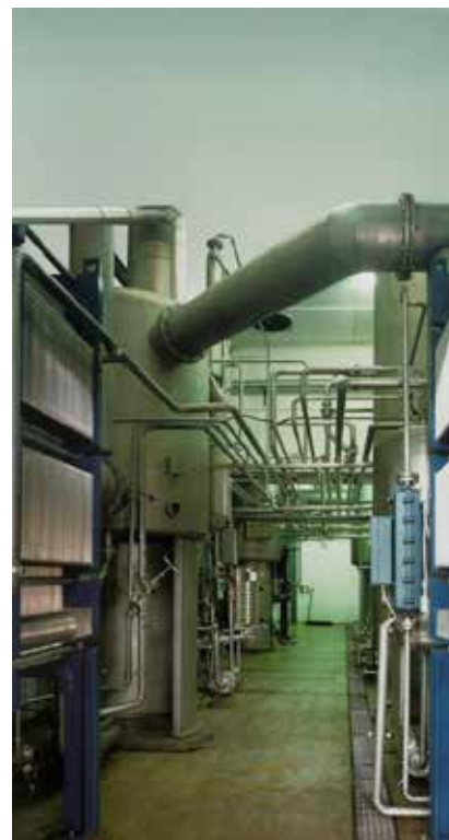
Installed Evaporation Plant
