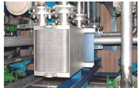
SIGMAWIG ST12 tempering of chemical reactor thermo-oil / ethylenglycol
